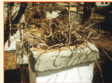
Look for the obvious! A blocked chimney cannot vent combustion gases out of the house.
