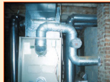
Horizontal vent runs must rise at least \frac{1}{4} inch per foot of run. The vent on this oil-fired furnace violates code and will never draft properly.
