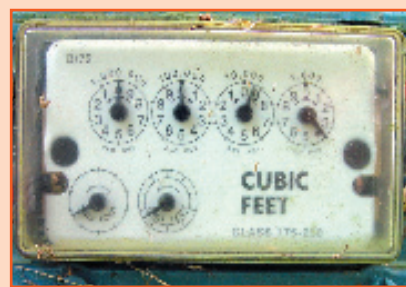
Most gas meters have 5 or 6 dials. Clock the dial that spins the fastest, which is the one labeled 1/2 or 1 cubic foot.
