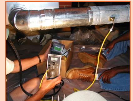
To measure CO in this floor furnace, the probe (not shown) is placed in each of the combustion ports. The draft probe is inserted in the vent as shown.
