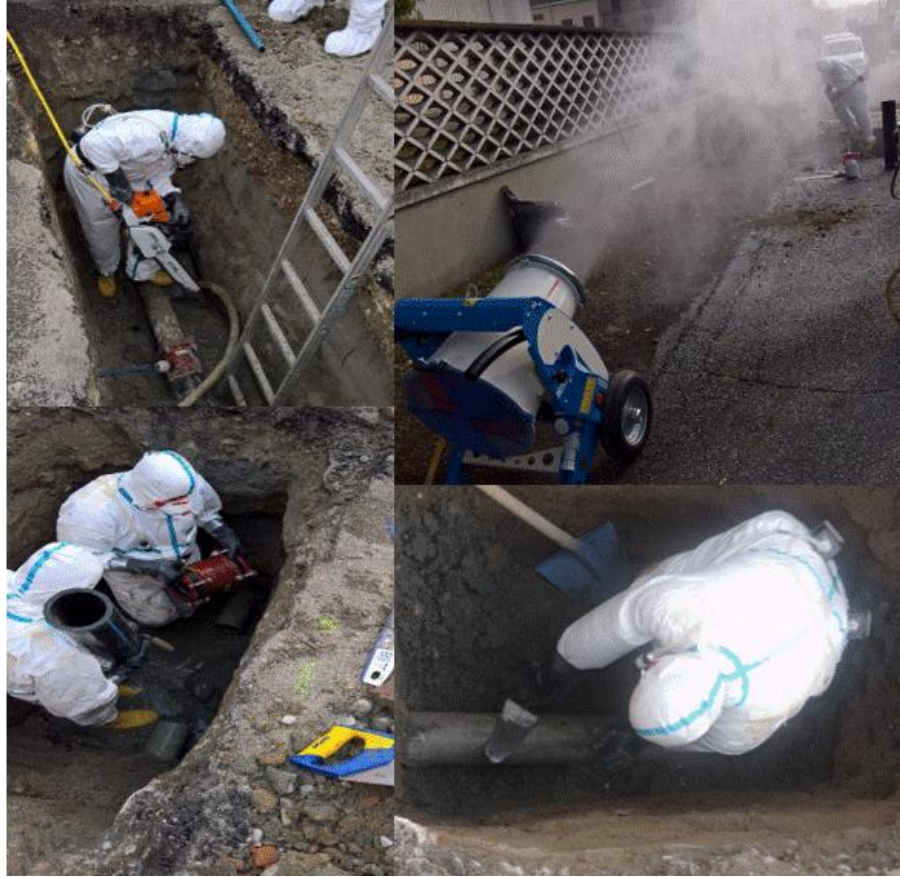
Fig. 3: Some examples of real cases some examples of real cases of interventions on asbestos cement pipes
