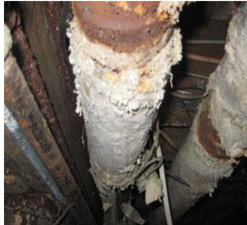
Figure 14. Pipe wrap is frequently hidden and may be difficult to find. Special wetting agents may be needed for pipe wrap.
