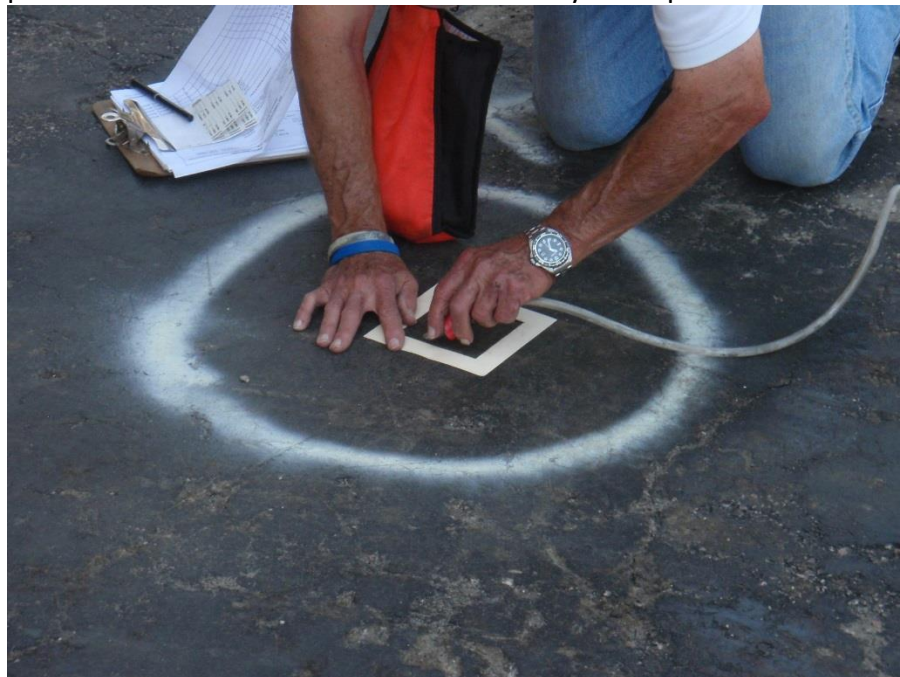
Figure 15. Micro-vac sampling is one method that may be used to indicate that non-porous surfaces, such as this asphalt parking lot, have not been contaminated by asbestos after the ordered demolition of the hotel featured in Figure 4. Photo courtesy of
