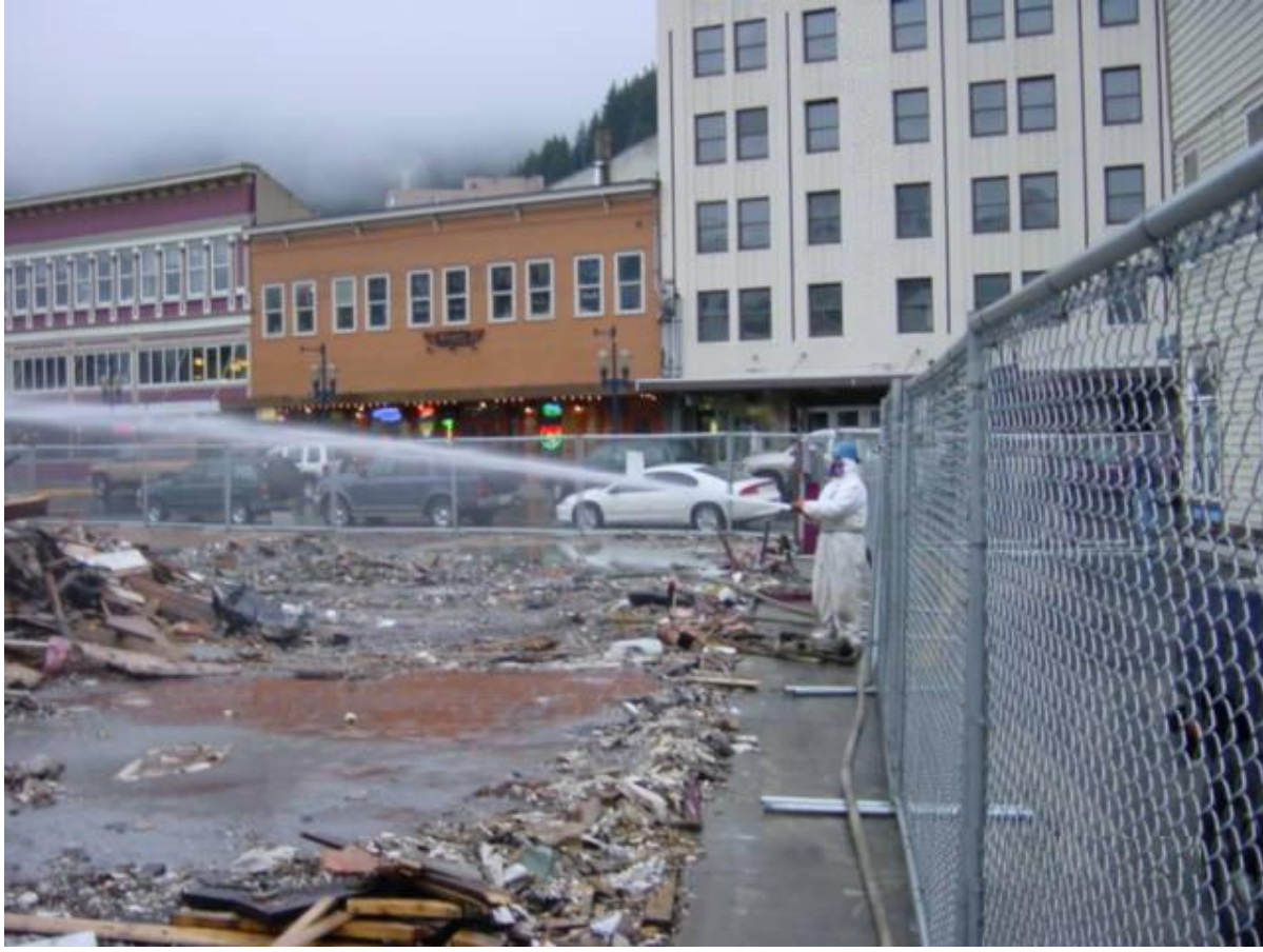
Figure 5. The surrounding sidewalk functions as a berm at this demolition, (EPA photo courtesy of John Pavitt, Region 10).
