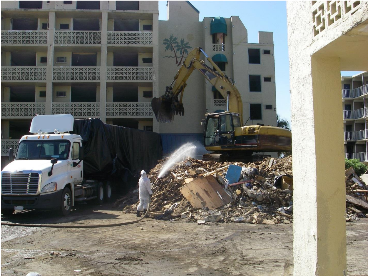
Figure 4. Ordered demolition of a structure on sandy soil in a coastal area. Water drains readily through this soil, and asbestos carried by the demolition water becomes embedded in the sandy soil. Photo courtesy of Pam McIlvaine, US EPA and Robin Mack, SCDEQ.
