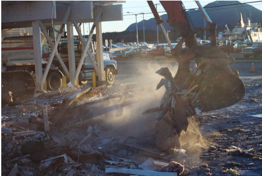
Figure 2. This photo illustrates the practical need for adequate wetting of asbestos contaminated materials. Dust containing asbestos is released when ACM are not removed prior to demolition. (EPA Photo courtesy of John Pavitt, Region 10).
