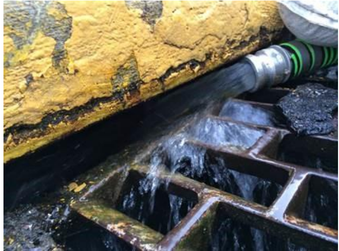
Figure 10. After filtration and testing of demolition water showed the water met effluent standards, it was released into the stormwater drain adjacent to the demolition project. Photo courtesy of John Pavitt, USEPA Region 10.
