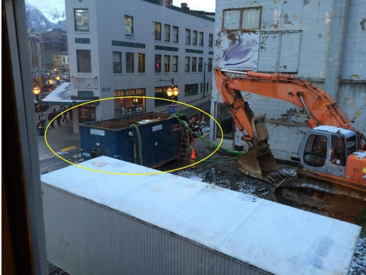
Figure 8. Water from a building demolition drained into the basement and was pumped to this tank (circled in picture) for settling before filtration to remove asbestos and other pollutants. Photo courtesy of John Pavitt, US EPA Region 10.
