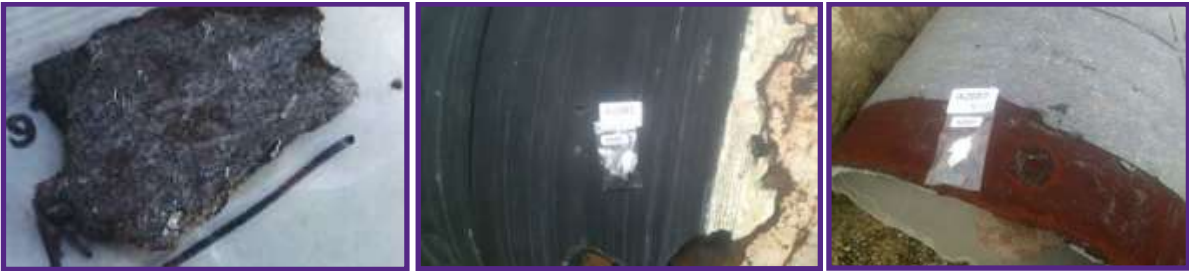
Figure 4.3: Coal tar or bituminous wrapped pipe pieces (on Water Corporation’s assets, these may contain asbestos and as such is treated as though it contains asbestos)
