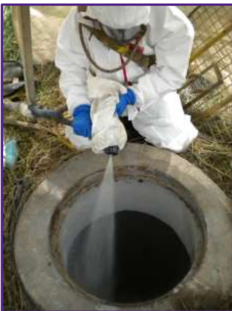
Figure 2.3: Manholes showing signs of deterioration being repaired. A special coating is applied to restore them to original condition.
