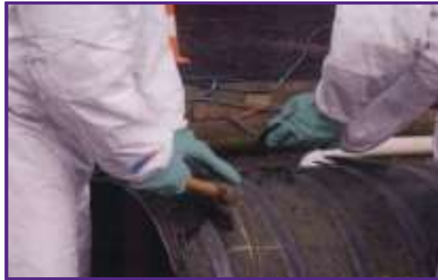
Figure 5.4: The hammer and chisel method used to remove asbestos from MSCL pipes
