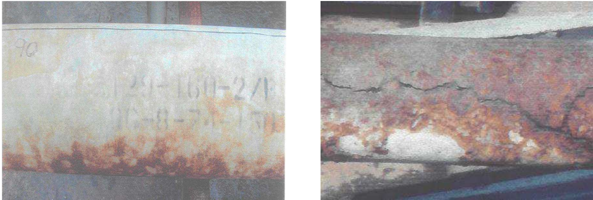
(a) Slightly deteriorated pipe
