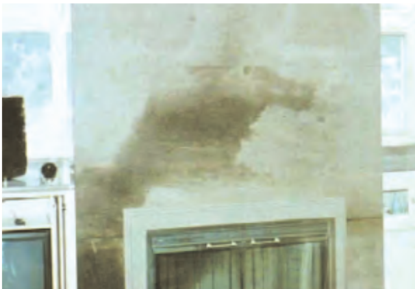
Wet stone on granite fireplace from a leak in chimney.
