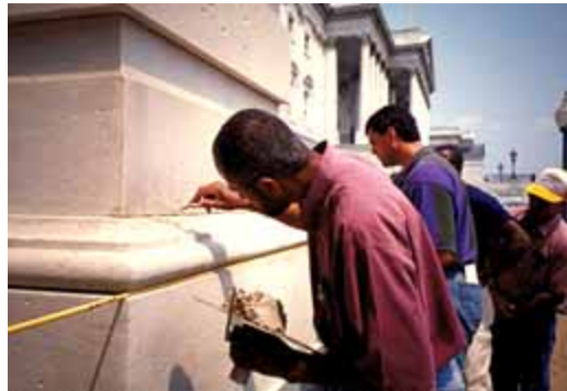
Masons practice using lime putty mortar to repair historic marble. Photo: NPS files.
