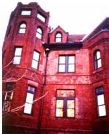
Unskilled repointing has negatively impacted the character of this late-19th century building. Photo: NPS files.
