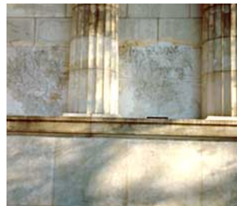
Damaging graffiti removal methods have scarred the marble. Photo: NPS files.
