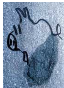
Poultice to remove pig graffiti. Photo: NPS files.
