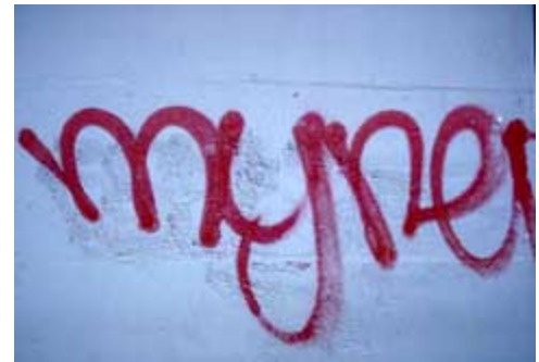
Inappropriate abrasive blasting to remove the graffiti has permanently etched the graffiti into the stone. Photo: NPS files.
