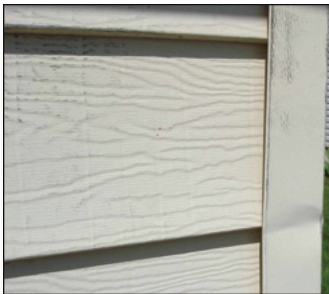
Figure 10—The corner of this house in Soda Springs, ID (Caribou-Targhee National Forest, Intermountain Region), is covered in steel siding that has been battered and bent over the years.
