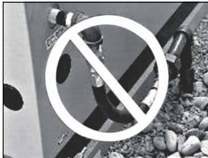
Figure 5-4. Incorrect Routing of Flexible Hose
