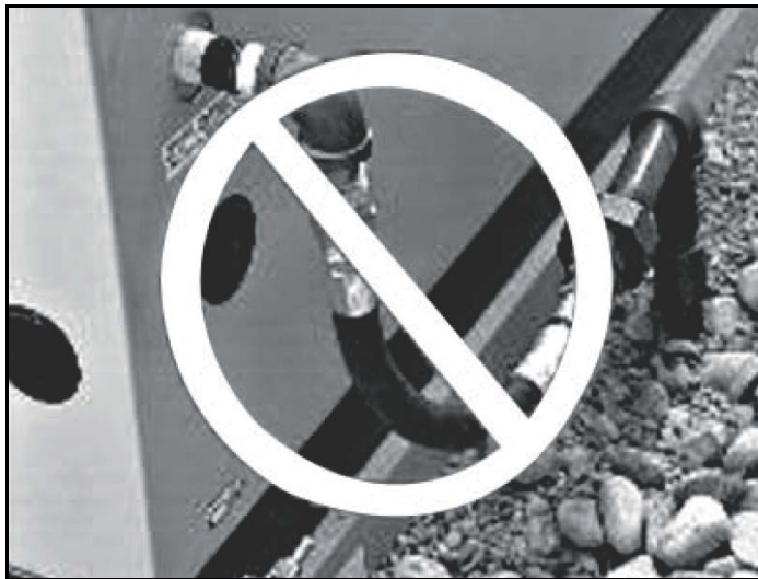
Figure 5-4. Incorrect Routing of Flexible Hose
