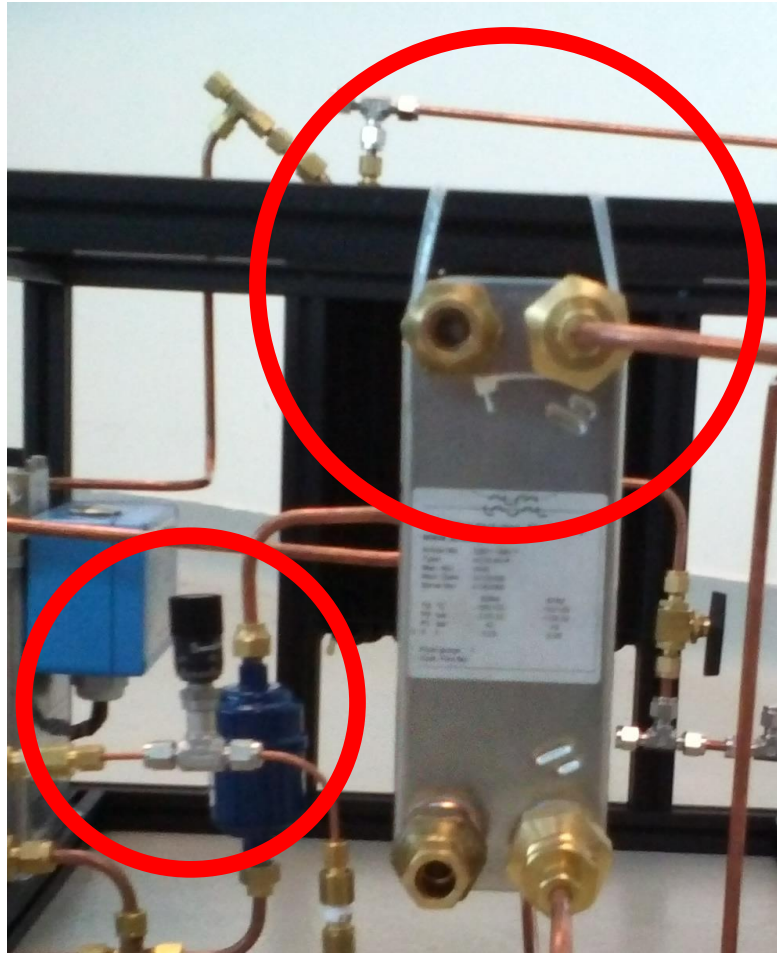
Figure 2.17: Wrong Installation for PHE and expansion valve
