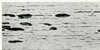
Fig. 22. Cracked or scaled paint such as this, resulting from the use of a low-grade product, must be removed before repainting.
