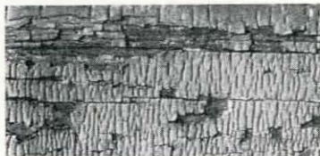
Fig. 13. Investigation of the formula before buying would avoid such results as these. Usually hard-type paints composed of cheap extenders and linseed oil substitutes fail like this.
