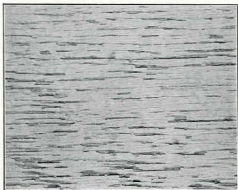
Fig. 46. Cracking and scaling.
