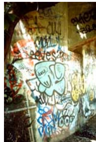
Removing this densely painted graffiti will require several applications of paint remover. Photo: NPS files.
