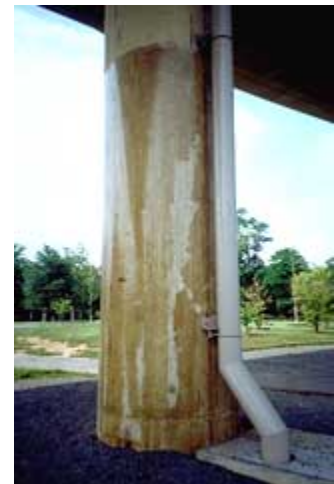
This formerly clear barrier coating is very shiny and has discolored as it has aged. Photo: NPS files.
