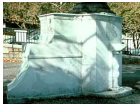
Painting over graffiti on stone is not a recommended maintenance treatment. Photo: NPS files.
