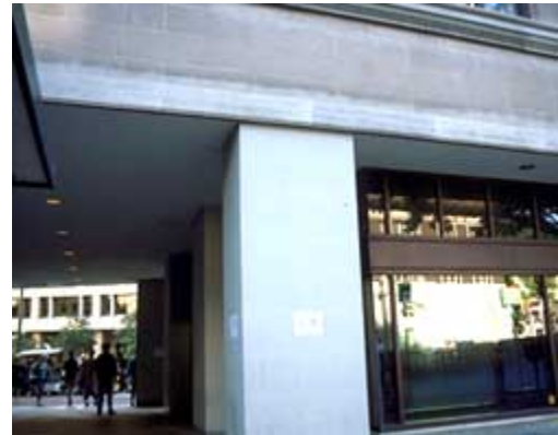
The difference in color between the bottom and the top of the stone spandrel is the only clue to the presence of a clear barrier coating. Photo: NPS files.
