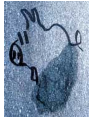
Poultice to remove pig graffiti. Photo: NPS files.
