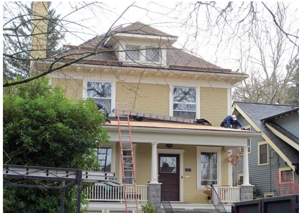
[16] The deteriorated asphalt shingles of this porch roof are being replaced in kind with matching shingles.
