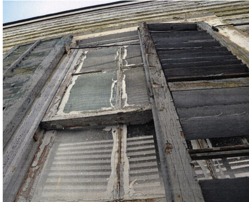
[11] Old and brittle glazing putty should be removed carefully before reputtying to keep window glazing weathertight.
