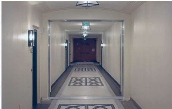
[58] Fire doors that retract into the walls have been installed here (not visible in photo) preserve the historic character of this corridor.
