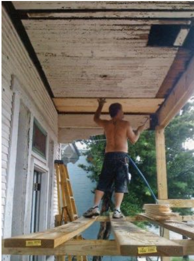
[24] Rotted boards in the beaded-board porch ceiling are being replaced with new matching beaded board.
