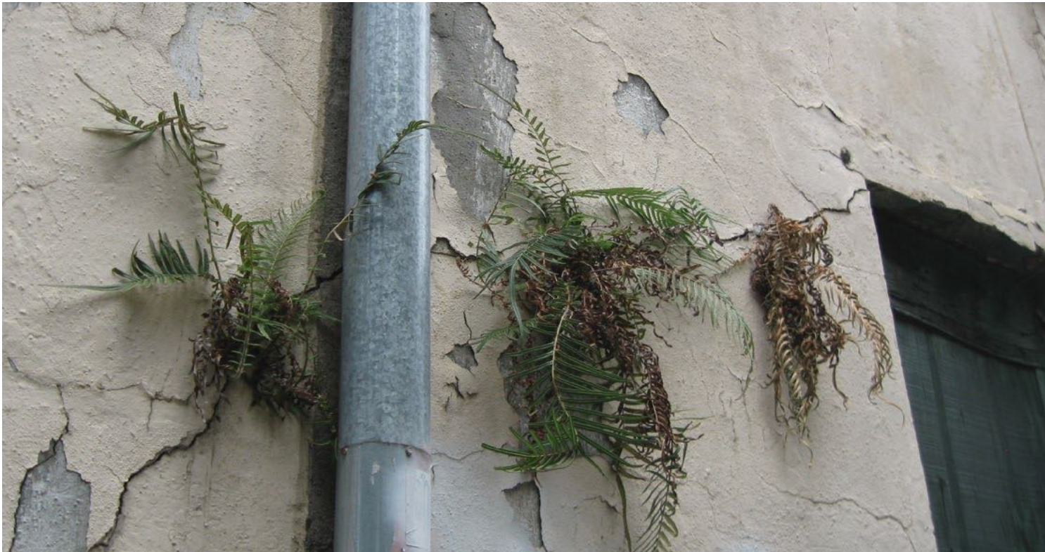
[3] Not Recommended: Cracks in the stucco have not been repaired, thereby allowing ferns to grow in the moist substrate which will cause further damage to the masonry.
