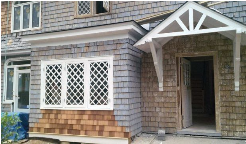
[5] Rotted wood shingles have been replaced in kind with matching wood shingles.
