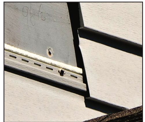
Figure 5. The siding panel was not properly locked into the panel below.
