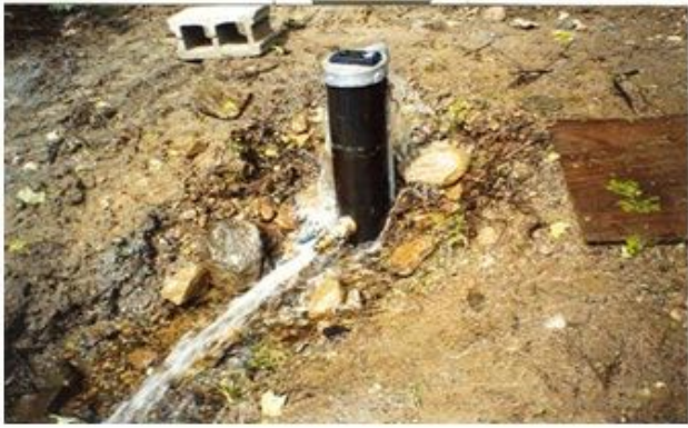
Figure 12-15 shows that if the valve is shut off, groundwater will overflow the well through the well cap. In this case, water is flowing out of the well even with the valve open.
