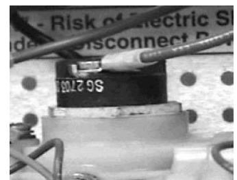
Figure 11: Installed heating element
