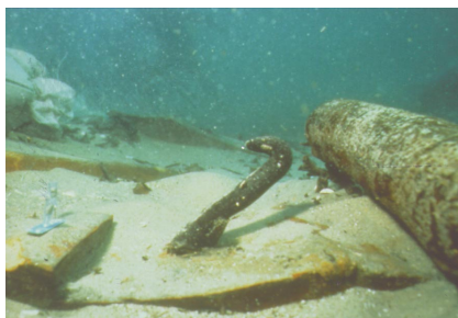
Figure 4. A metal nail still attached to a floor timber after removing the futtock.
