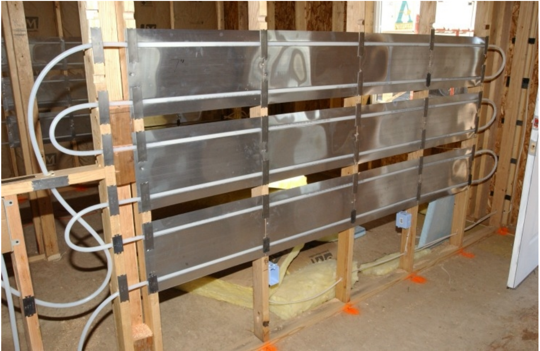
📷 In-wall radiant heating in a house under construction near Denver. | Photo courtesy of Warren Gretz, NREL.
