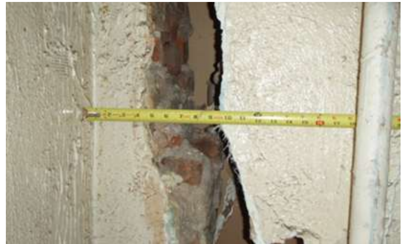
Interior cracks on wall perpendicular to bulge
