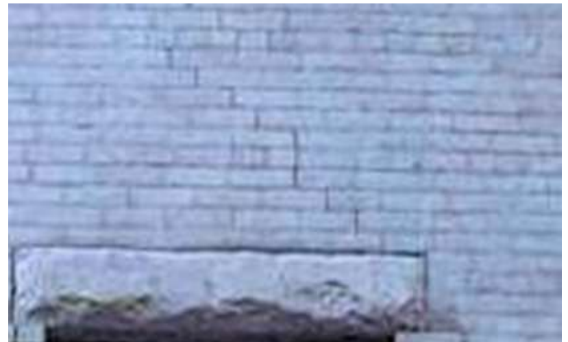
Unrepaired Stepped Crack
