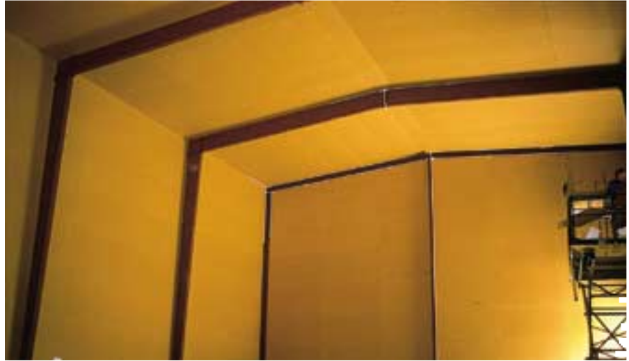
MDO panels are applied to the interior of a cold storage building.
