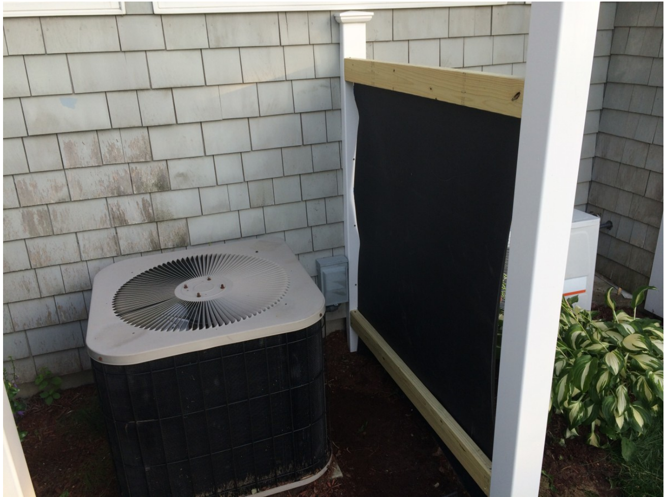
Inside AC Enclosure
