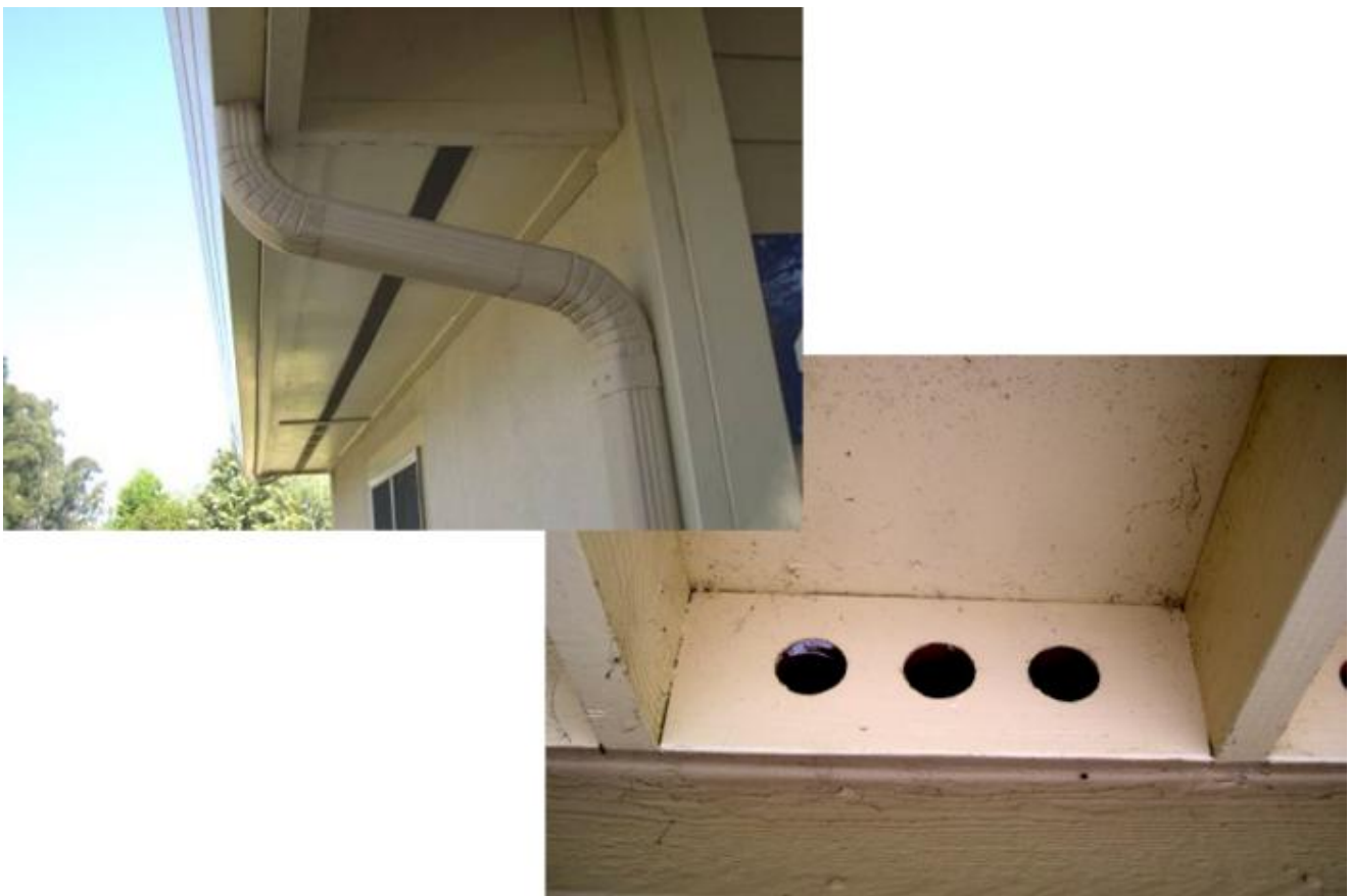
Vents are vulnerable to wildfires when embers and flames enter into the enclosed attic or crawl spaces, and ignite combustible materials in those areas.
