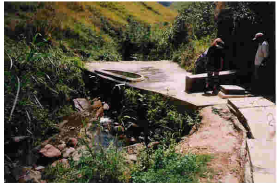
Spring box with roughing filter on the outlet (to the right) prior to the water entering the pipeline
