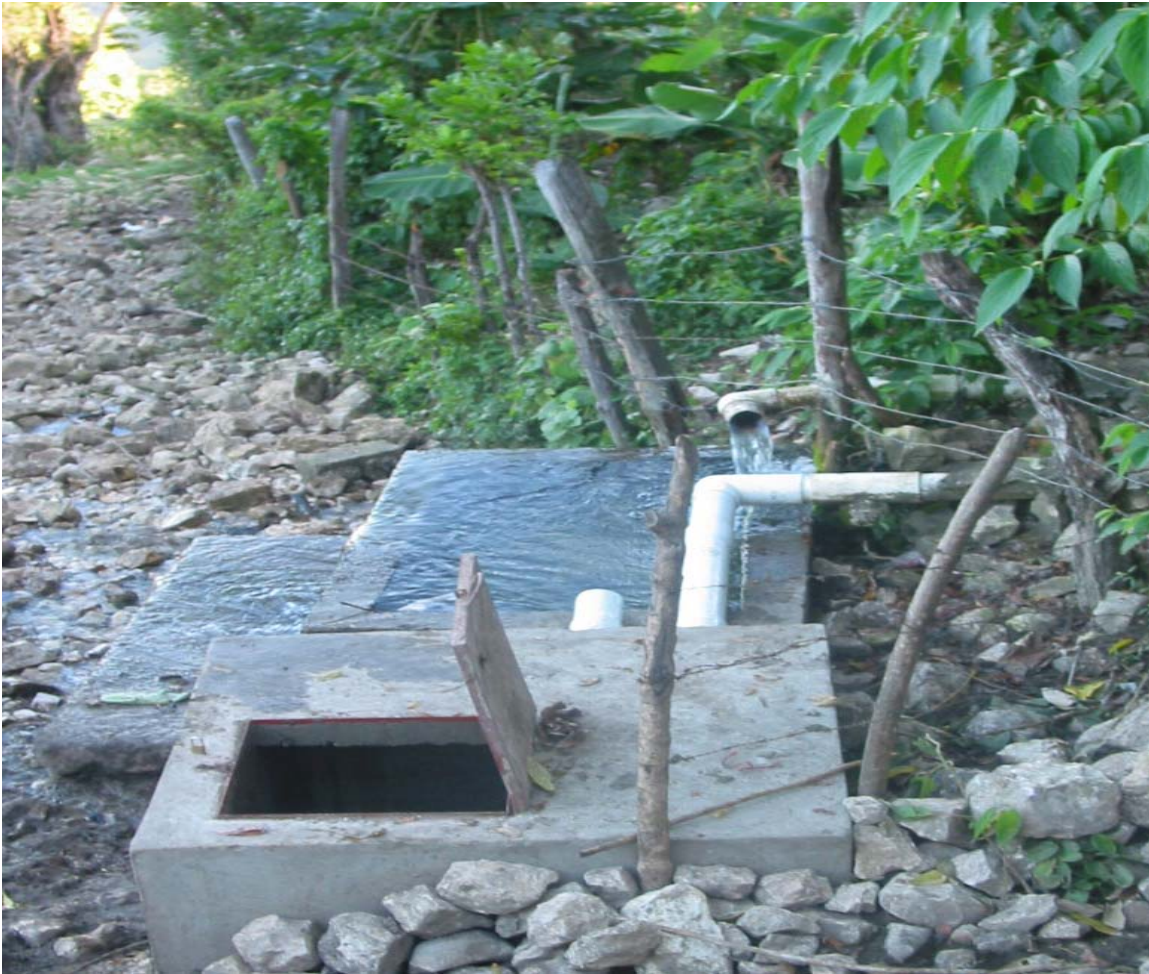
A newly completed spring box in the Dominican Republic. Note old spring box behind the new structure with open top to allow livestock a drink of water. Photo courtesy of Matt Niskanen, 2003.
