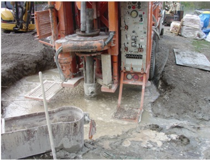
Figure 12-6 shows the back of an orange coloured drilling rig. A black coloured drilled well casing extends out of the muddy water through a rotary table. The drilling rig is holding on to the casing with the rotary table and a welded piece of steel. During drilling the flow around the outside of the casing created a void in the ground. The overburden above the void has collapsed creating a 10 metre (30 foot) deep by 4 metre (13 foot) wide hole filled with water. The void was unknown until the time of overburden collapse. The void created a serious safety issue for anyone working on the back of the drilling rig.
