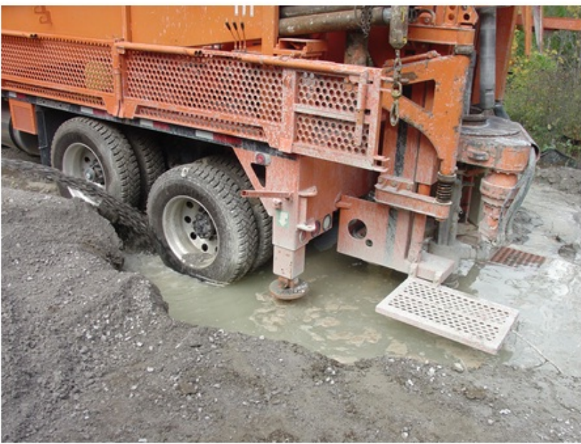
Figure 12-7 shows the same drilling rig and void shown in Figure 12-6. The drilling rig is slowly falling into the hole jeopardizing the drilling rig. In this case, the well contractor took immediate measures to fill the void and rescued the drilling rig.
