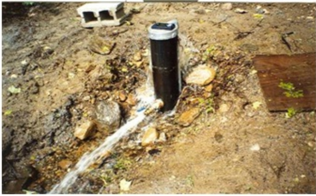
Figure 12-15 shows that if the valve is shut off, groundwater will overflow the well through the well cap. In this case, water is flowing out of the well even with the valve open.
