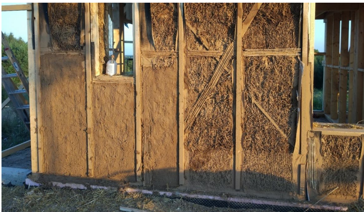
Figure 7. Exterior wall in the process of being plastered with clay. Photo: Michał Pierzchalski.
