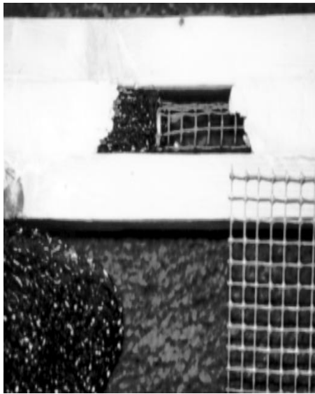
Fig. 9. Patching small holes with copper gauze and a fast-drying patching compound (left), and 1/4-inch hardware cloth for larger holes (right).
