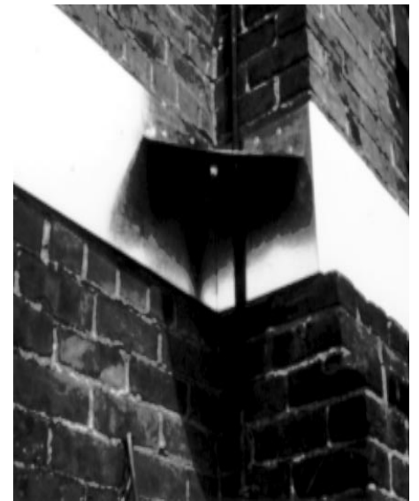
Fig. 20. Sheet metal band attached to outside walls to prevent rodent climbing. Band should be 14 to 18 inches wide and 30 inches above where a rodent can jump from.
