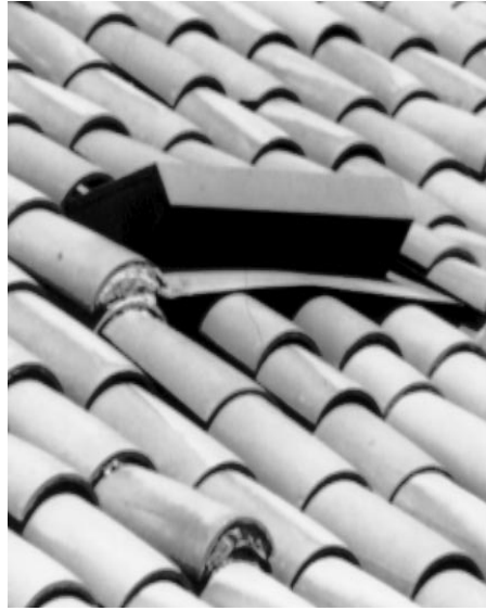
Fig. 6. Poorly installed light-gauge roof vent, allowing easy access of rodents between roofing and base of vent. Gaps were large enough to allow rats and pigeons to enter.
