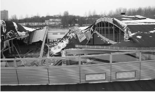
Fig. 1. The Siemens arena roof structure after the collapse of two trusses. An intact truss can be seen on the right.
