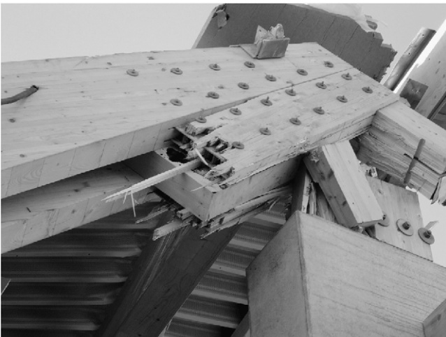
Fig. 3. Rupture at the critical cross-section in the corner connection. Note the dowels and steel plates.
