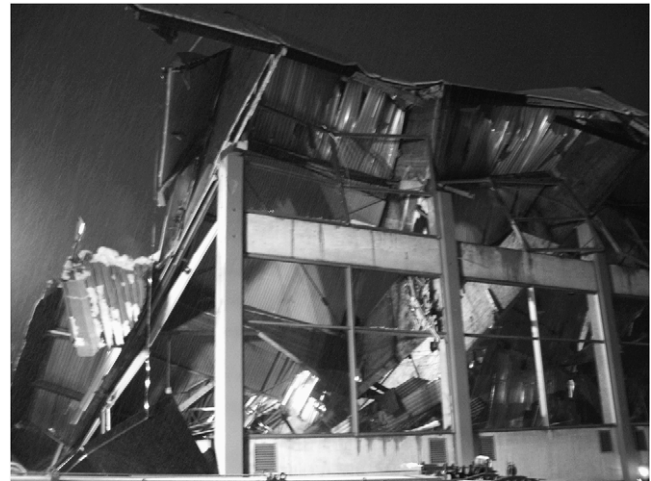
Fig. 5. Partial view of the collapsed roof structure.
