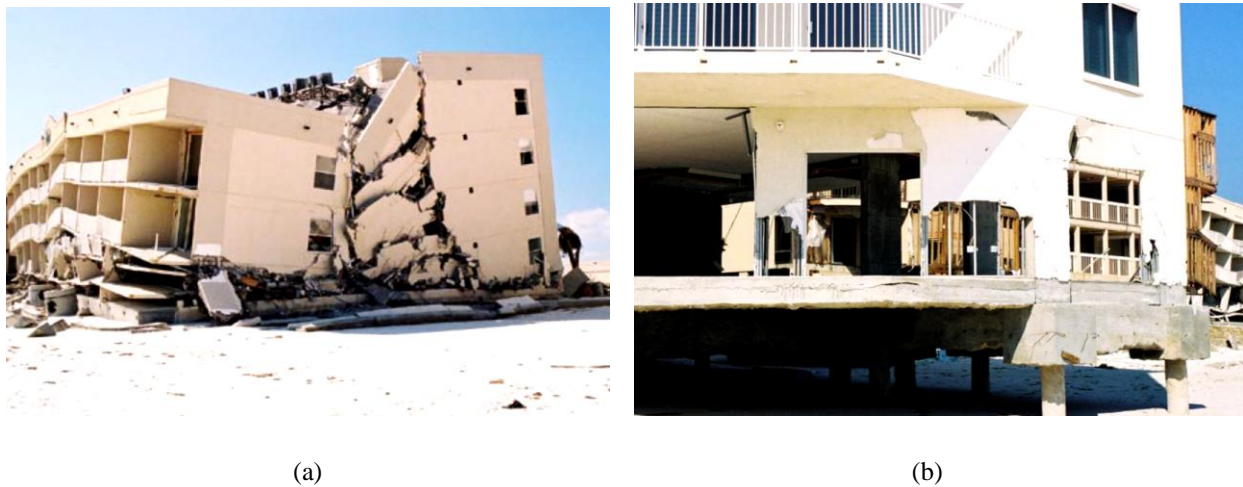
Figure 11. Several flood-induced damage to concrete buildings during Hurricane Ivan, 2004 (FEMA P-550): (a) severe structural damage to the building with shallow foundation due to surge, wave, and floodborne debris; (b) partial/complete collapse of exterior walls below the BFE for a concrete building elevated on deep piles.
