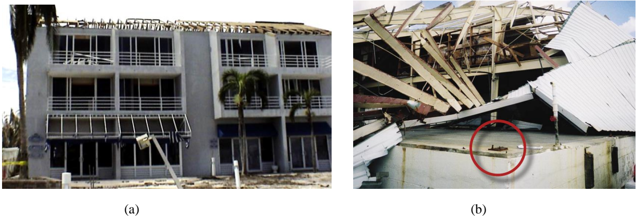
Figure 10. Wind-induced damage to concrete and steel frame buildings during Hurricane Charley, 2004 (FEMA P-488): (a) damage to a multi-family building roof deck with inadequately supported and braced overhang; (b) roof framing failure and gable end wall collapse due to insufficient lateral supports.
