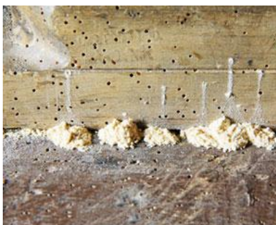
Powderpost beetle exit holes and accumulated sawdust (Photo: townandcountrysolutions.com)
