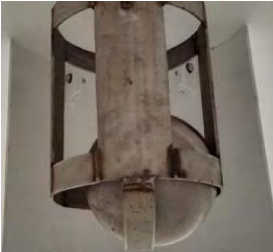
Primary Shutoff Assembly (Collection Tank Interior)
