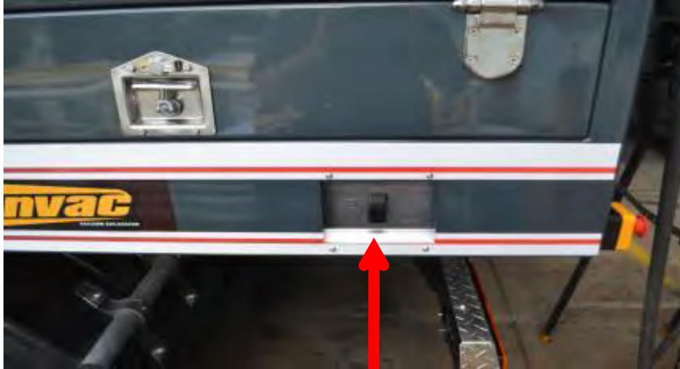
Water pump Switch
