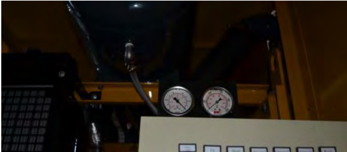
Blower Pressure/Vacuum Gauge
