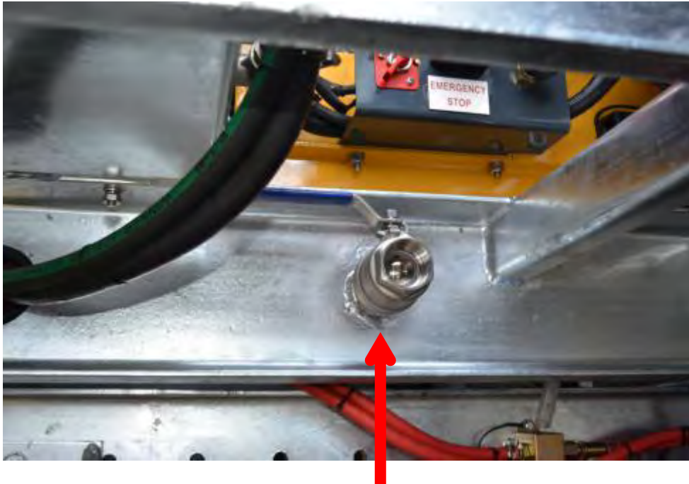
Water Tank Drain Valve Lever
