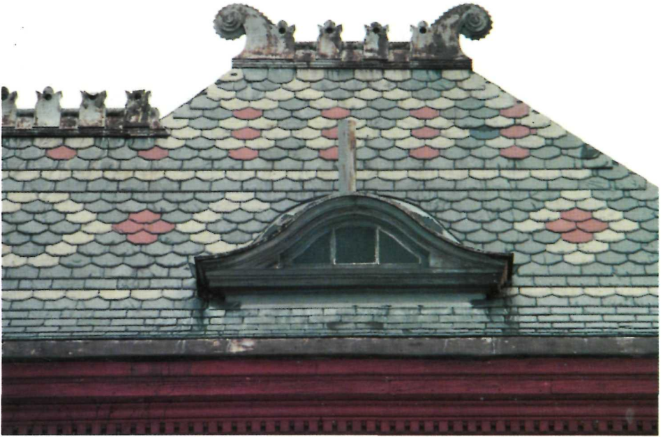
85* Base flashing above eyebrow window and cap or counter flashing below. Note also rusting galvanized iron ridge pieces
