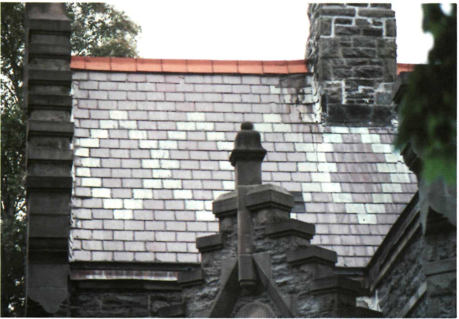
89* Problems with a terracotta tile ridge, Park Lodge, Halifax
