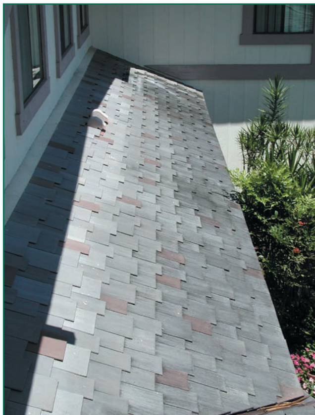
Photo 4 – Blackish algae growth begins below eave-protected, shaded area
