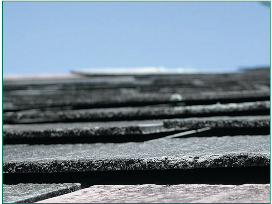
Photo 3 – Crumbling deterioration at leading edge
