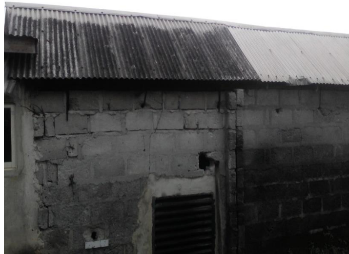
Fig. 1. Building in Uyo Metropolis: The Roof is Completely Covered with Dark-Black Deposit.
