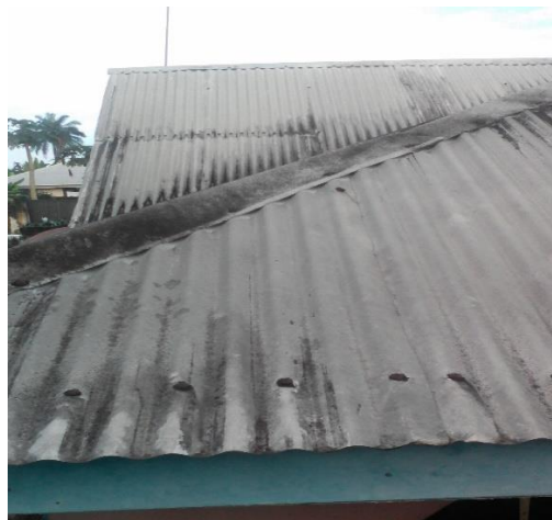
Fig. 3. Building Roof Completely Covered with Dark-Black Deposit.
