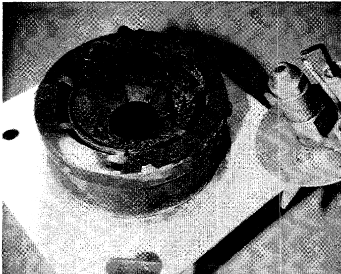
WET-BASE BOILER 1.75 GPH COLORADO FUEL
