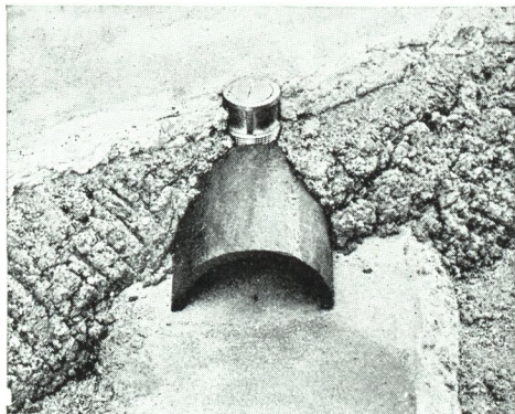
Showing installation of Orangeburg System of Underfloor Duct in a floor of over 3" fill. Note "pad" or "bench" provided under duct and inconspicuous floor outlet.
