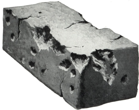
This illustration shows how severe heat attacks and destroys fire brick when it is not properly protected by carefully chosen refractories. Surface cracking and spawling and the expense of consequent shut downs and replacements, can be reduced by bonding and wash-coating fire brick with Johns-Manville refractories.
