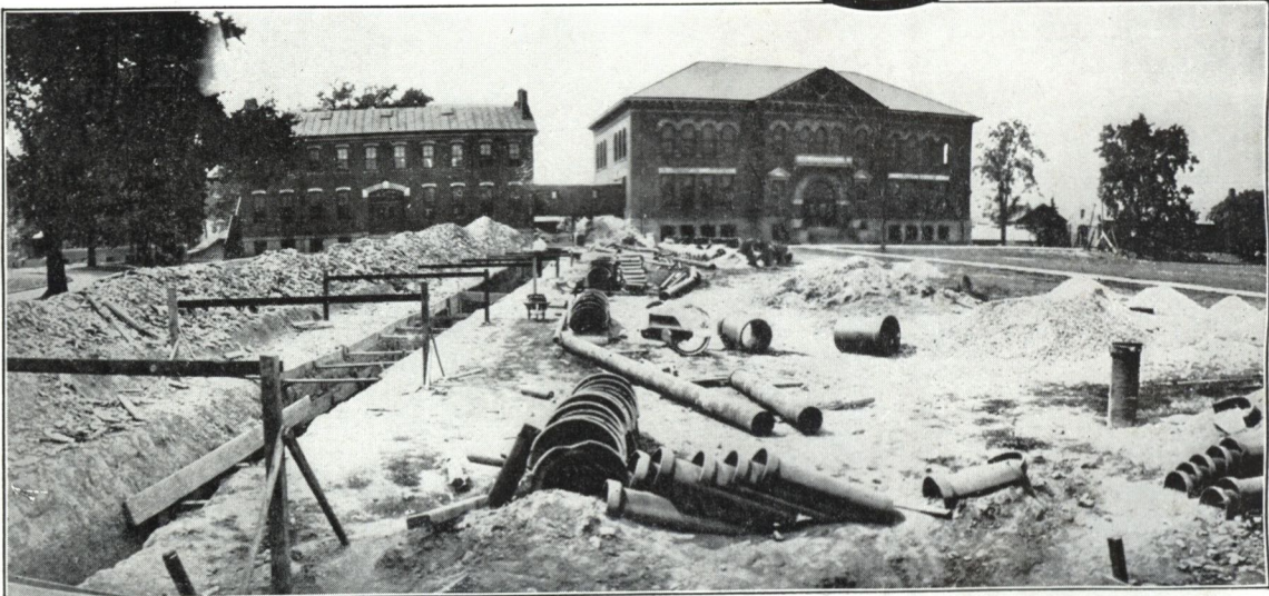
Sections being split before being placed in trench at Pennsylvania Reform School, Morgantza, Pa.
