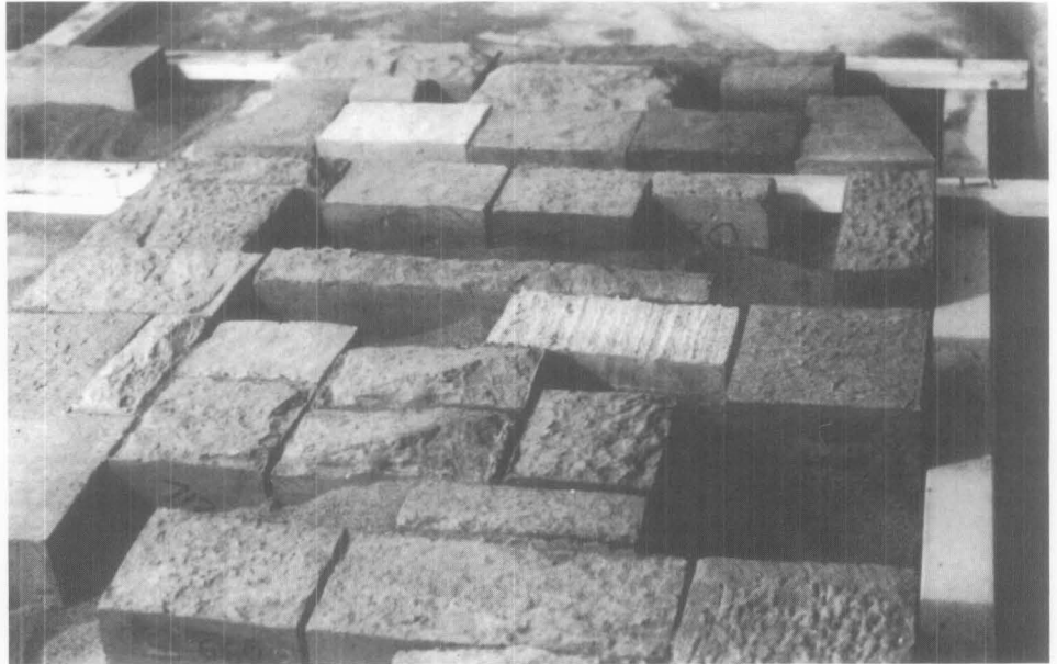
Figure 9. Using the measured drawings as a guide, the pre-cast units were assembled in the staging area on top of 4 inches of sand prior to their installation on the facade. Photo: Robert Powers
