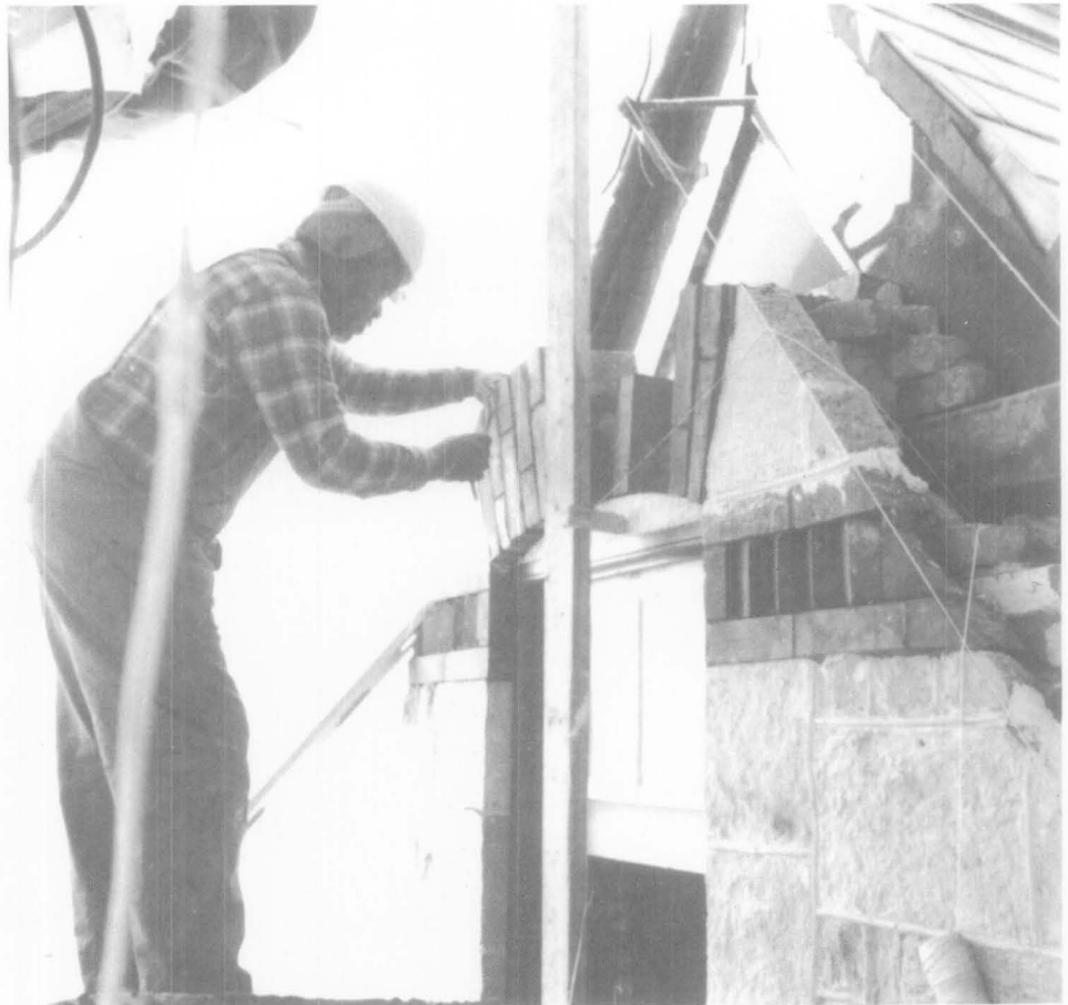
Figure 10. The new pre-cast units were hoisted up the scaffolding on wide belt slings with an electric winch, and installed in place using a portland cement-based mortar appropriate for cast-concrete. The original bricks were relaid with a more traditional lime-based, dark-colored mortar. Photo: James Smith
