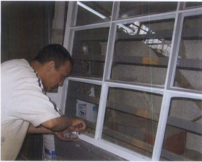
Figure 6. The outer glass was installed in the traditional manner, using exterior glazing putty. Photo: Charles Fisher.
