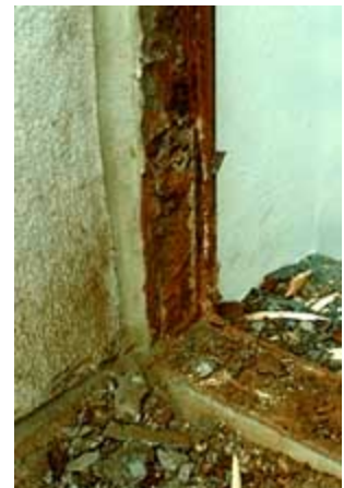
A severely deteriorated frame, such as this, can be replaced in kind.
