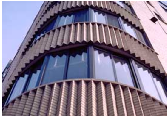
The historic steel sash (see photo above) was removed and replaced with modern aluminum sash, resulting in a negative visual impact on the building's historic character. Photo: NPS files.
