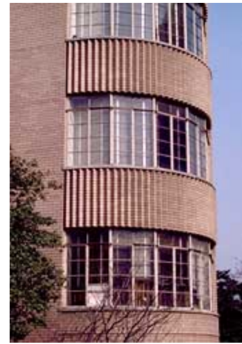
The historic steel sash is shown in place, prior to its removal and replacement with inappropriate aluminum sash (see below). Photo: NPS files.
