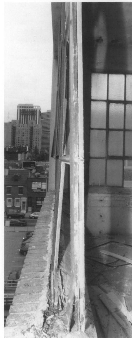
Figure 8. Bowed and corroded window during construction. Photo: Clío Group.
