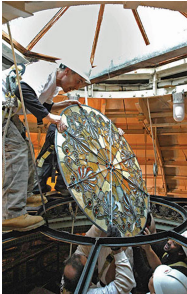
(b) Workers install a jeweled art glass oculus of a Healy & Millet dome. The diffusing skylight was restored overhead to reintroduce daylight to the historic 1897 dome after being roofed over since the 1940s.
