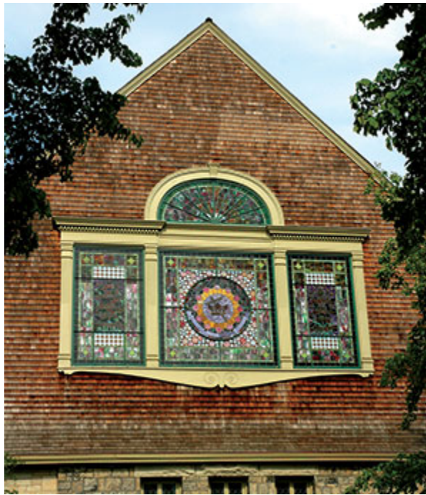
Figure 5. Stained glass is an exterior feature as well as an interior one. As part of any preservation project, stained glass should be photographed from the exterior as well as the interior.
