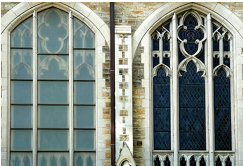
Figure 18. On this pair of neo-gothic church windows, the aluminum frame grid used for protective glazing disregards the original tracery of the window on the left. The grid mars the appearance of the window inside and out. It also impairs the overall historic character of the building. The plastic storm glazing has been removed from the adjacent window to restore the original window appearance.
