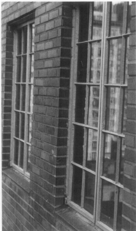
Figure 7. The dark frame color and careful installation of the interior storm window resulted in little visual impact on the exterior appearance of the building. Photo: Charles Fisher.
