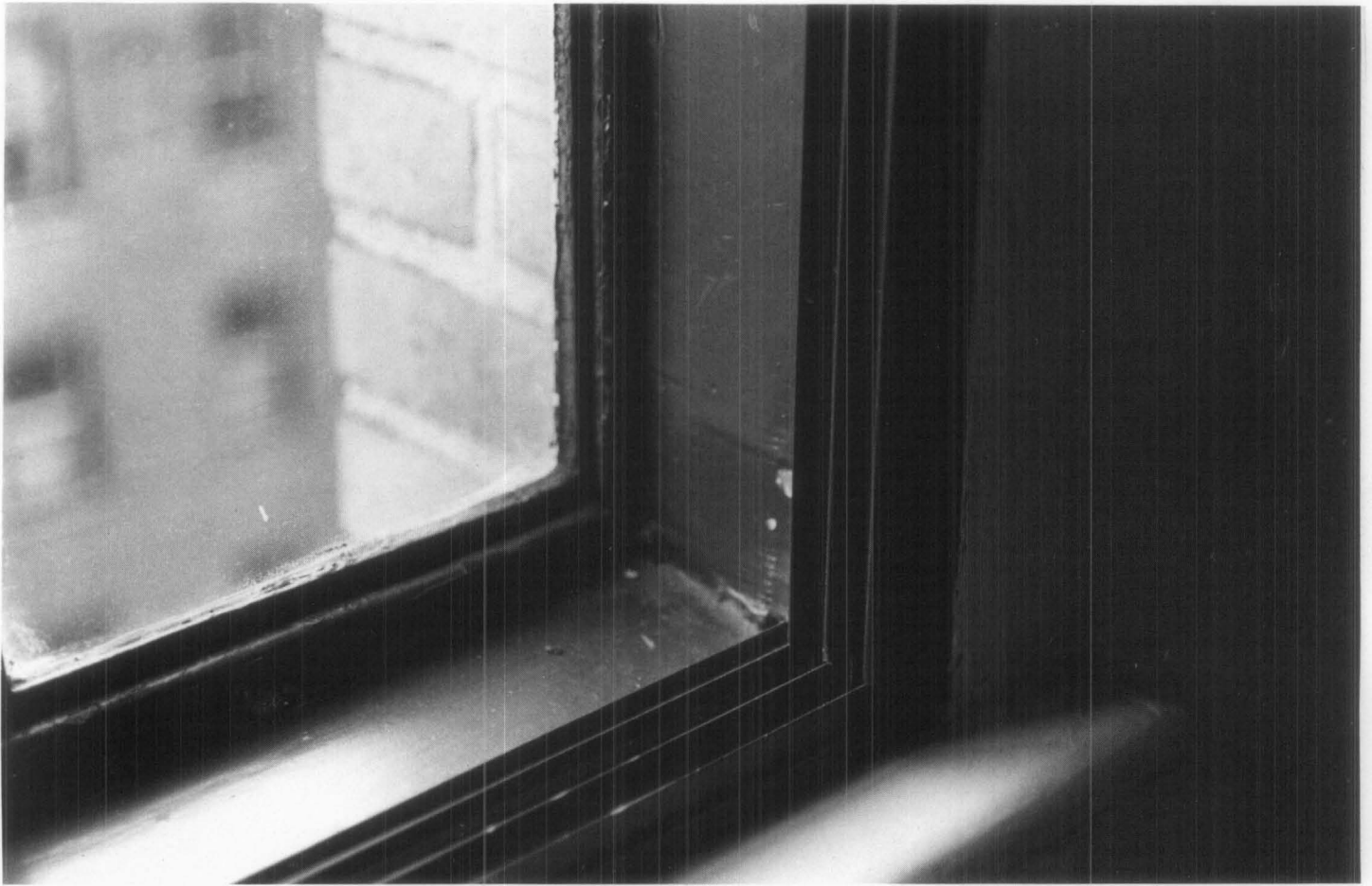
Figure 6. The subframe had to be squared off when installed in each window opening to prevent racking of the sliding panels. Photo: Christina Henry.
