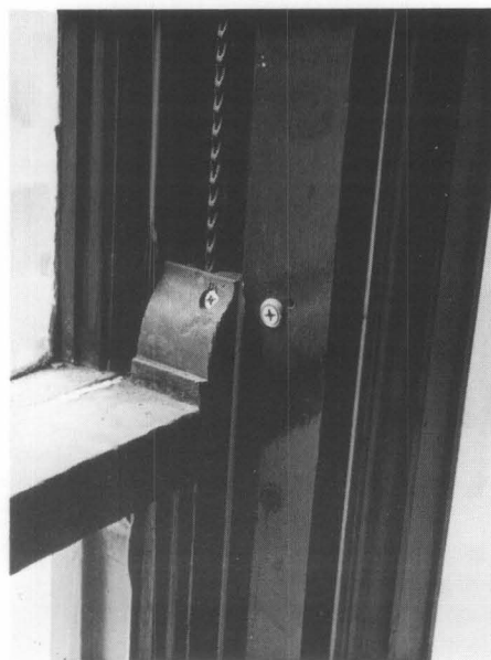
Figure 4. The only modification made to the windows was the addition of a screw through the decorative end of the sash stile to fix closed the operable portions. This decision grew out of the recommendations by the mechanical engineers. Photo: Charles E. Fisher
