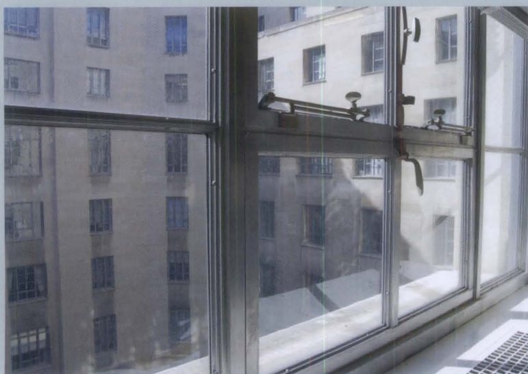
Figure c. In cleaning historic aluminum windows, the gentlest means possible should be used. More aggressive cleaners should be used only where necessary. The interior surface of this window was cleaned ten years ago with an aluminum jelly cleaner, rinsed and then dried thoroughly. The original mill finish still retains its luster.
