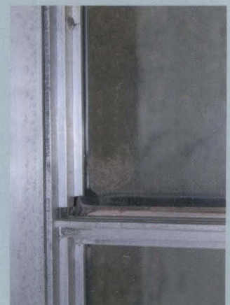
Figure b. The panes of glass were secured into the frame with aluminum glazing stops, each individually cut, drilled, and fixed in place from the inside. Here the vertical stop is in place while the horizontal is missing.
