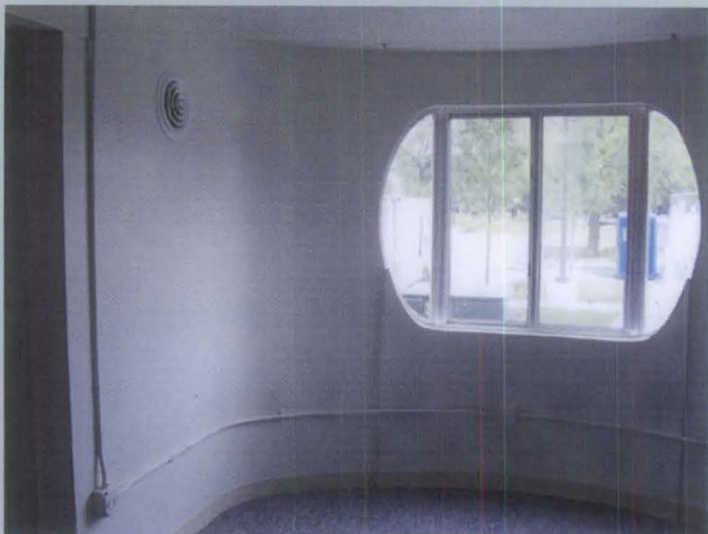
Figure e. Both interior and exterior aluminum surfaces had become dull, soiled, and oxidized as a result of traffic exhaust and air pollution. Cleaning the aluminum stabilized any further deterioration and brought back the luster of the original mill finish. (Photo: Holsten Real Estate Development Corp.)
