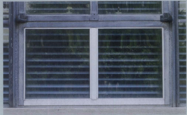
Figure d. Numerous hopper units have been removed over time to accommodate air conditioning units. Replacement hopper units were manufactured, as needed, to match the original hoppers elsewhere in the building.
