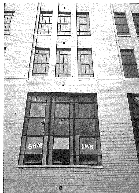
Figure 4. Among the retained and repaired original windows were these large units on the second floor level. Photo: Bruner/Cott & Assoc., Inc.
