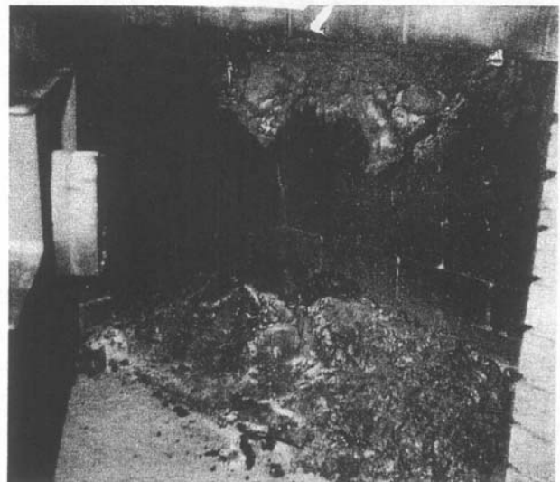
Figure 2-8. The aftermath of a chimney fire is marked by a large quantity of pyrolyzed creosote residue in highly expanded form. Ash is six or more inches deep on the firebox floor and a large mass is hanging from the fireplace damper area.
