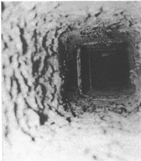
Figure 4-2. Looking down into a chimney lined with clay flue tiles after a chimney fire. Note that the lower tiles have been burned absolutely clean while the higher tiles show significant amounts of expanded creosote ash. Close inspection reveals cracks in the liner, but no liners are displaced.
