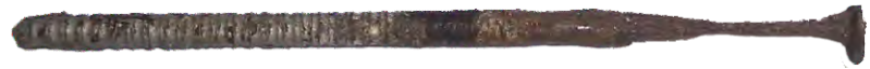
Example of a severely corroded electrogalvanized fastener. Ensure the correct fasteners are used. Corroded fasteners lead to serious sidewall system failures as well as unsightly staining.
